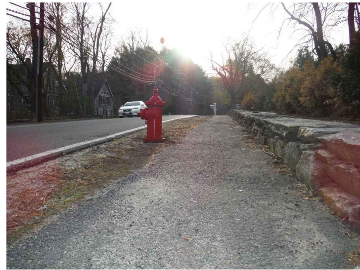
EXISTING SIDEWALK LOWER THAN ROADWAY
