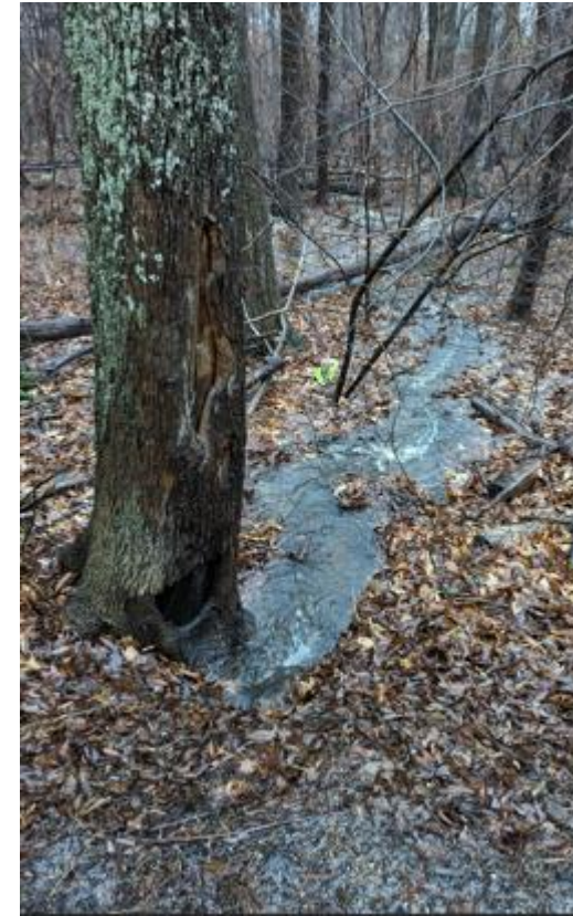
Other side of Parkerville at Culvert Outlet
